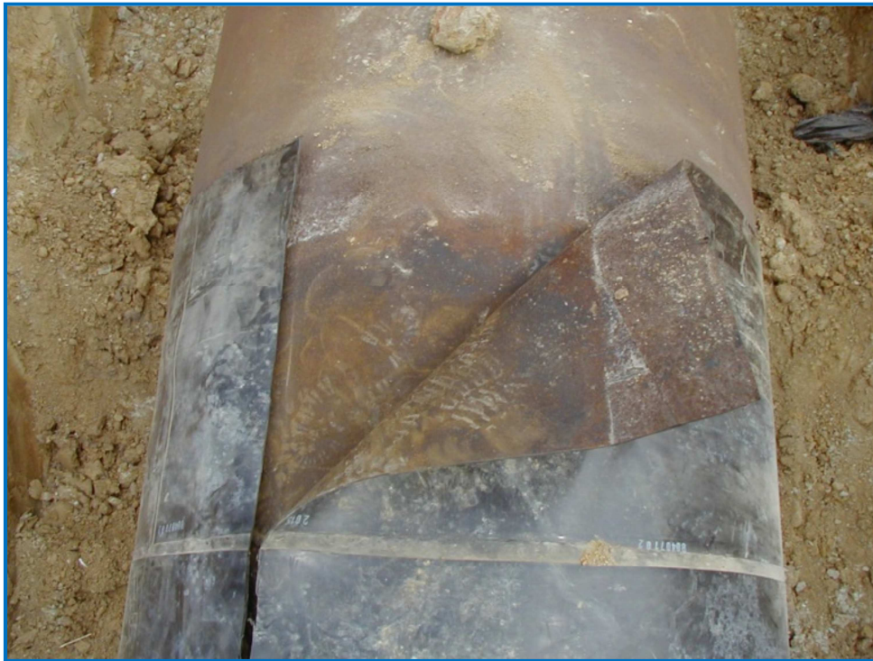
Figure 6.48 Conditions of the rehab shrink cuff after several years of operation
