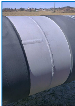
Figure 6.49 Transversal weld, prepared for insulation (DN 800, 3LPE, surface preparation level Sa 2½ - EN ISO 8501-1)
