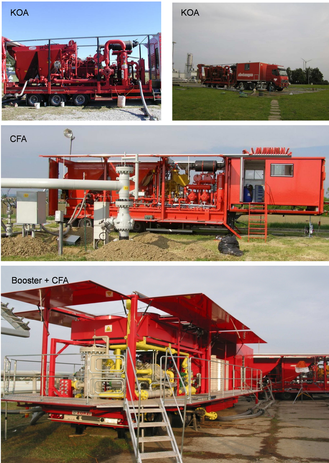
Figure 6.12 Compressors used by Eustream + booster unit
